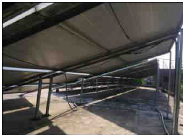
Figure 3.10: Power cables lying unclipped can result in serious incidents and fire hazards.
