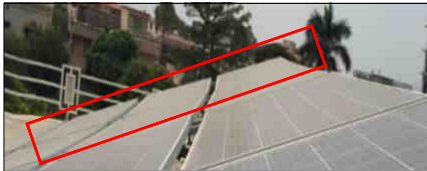
Figure 3.14: The string highlighted in the picture is convexed due to inappropriate mounting structure
