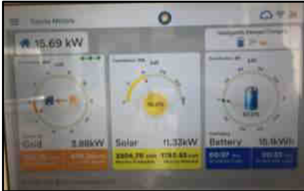
Advanced SCADA-based HMI (Human to Machine Interference) for data recording, monitoring and control.
