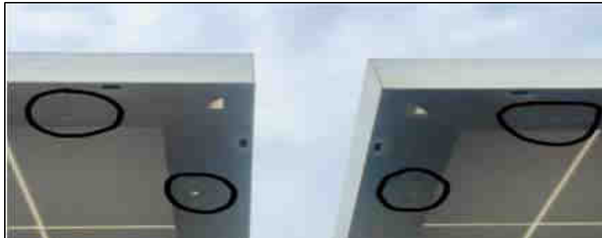
Figure 3.12: The proper grounding procedures for earth connectivity needs the PV panels to be connected electrically.
