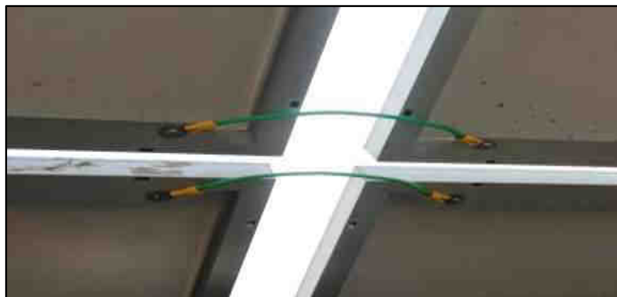
Figure 3.13: The panel-to-panel electrical connection of the module's frame is recommended for compliance of the standards.
