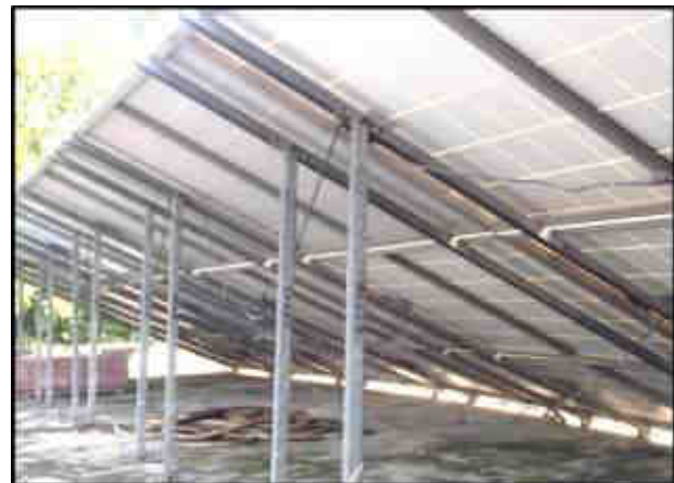
Figure 3.11: The inadequacy in wiring and cabling when PV module is connected in strings.
